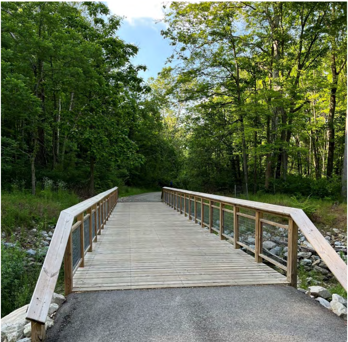
Cleveland Metroparks pedestrian bridge at the North Chagrin Reservations' Wilson Mills Trail Head. CT Consultants.
